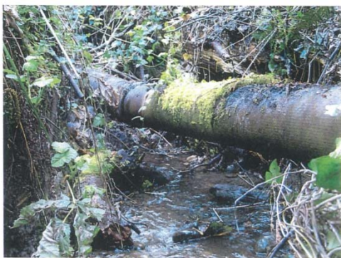
Exposed sewer line in watercourse (before)
